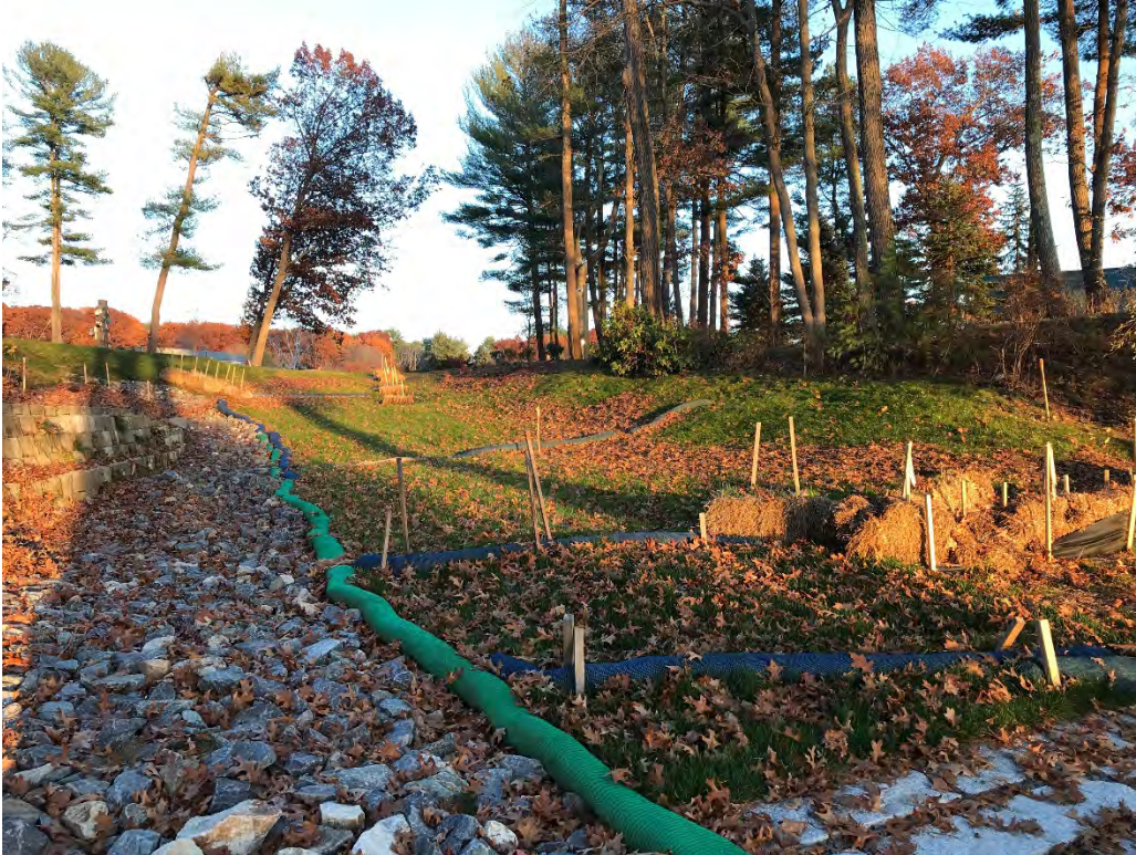
Fig 3: Slope above the manhole at Gundalow Landing/east side of the bay. Viewing east. (11-10-20)
