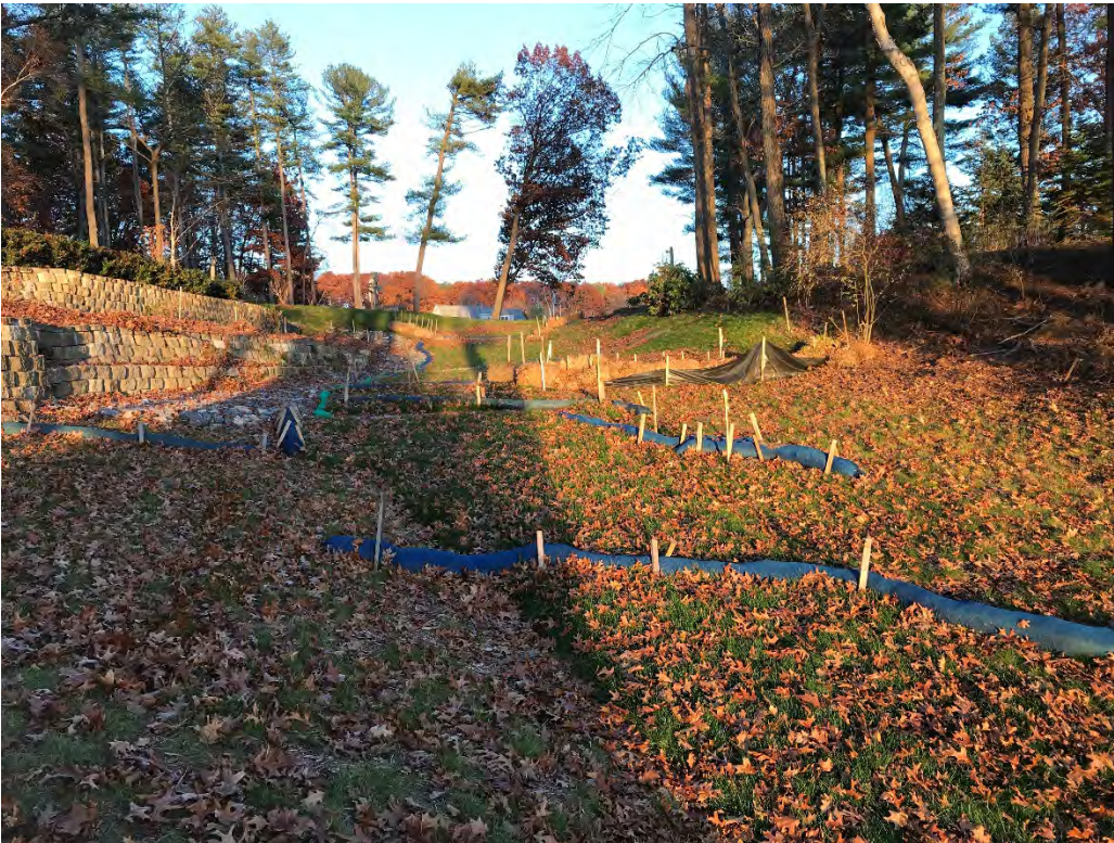
Fig 4: Slope below the manhole at Gundalow Landing/east side of the bay. Viewing east. (11-10-20)
