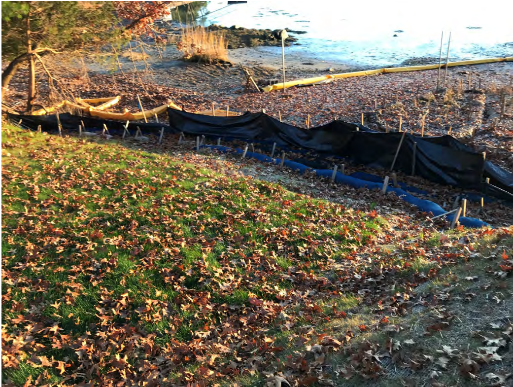
Fig 5: Toe of the slope at Gundalow Landing/east side of the bay. Viewing south. (11-10-20)
